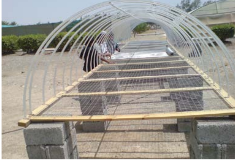
(b) Tunnel placed on concrete block substructures showing dryer part without wooden base over the metallic net
